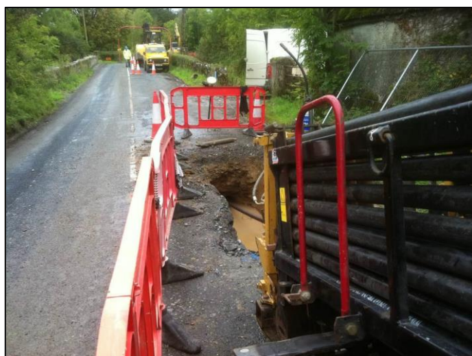
Figure 2-26: Standard HDD site on local road where HDD was used to go underneath a bridge (bridge parapet walls visible).
