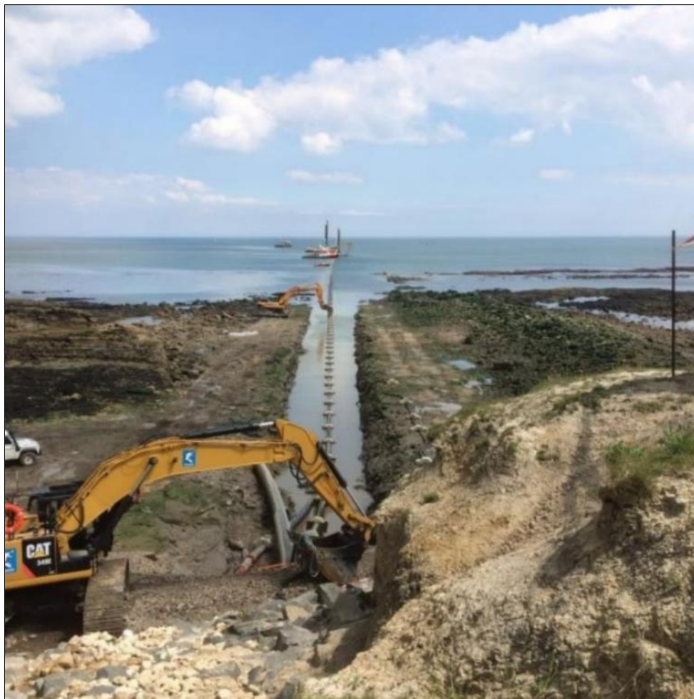
Figure 2-13: Photo showing installation of a cable in a trench at a landfall.
