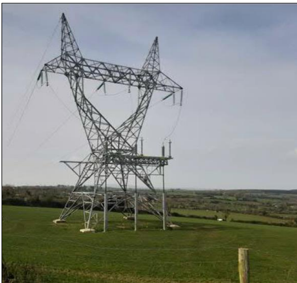
Figure 2-29: Photo of 220 kV Line Cable Interface Mast with shield-wire facility.
